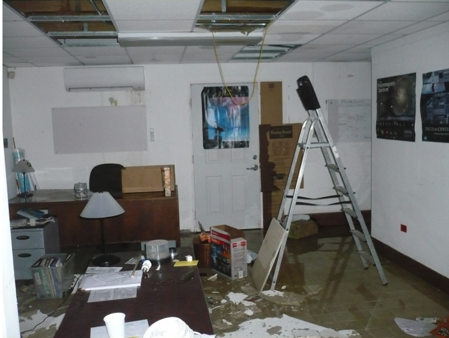
Fig. 5. Picture of the control room taken after the hurricane Irma, and before the hurricane Maria. The computers were stored in a safe place; it is however clear from the picture a lot of work is due before the operations can resume at the Observatory.
