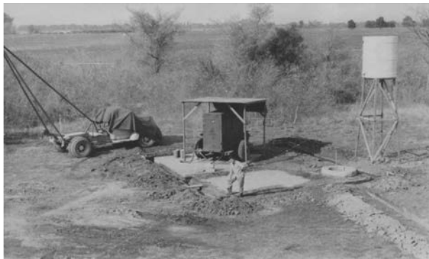
Fig. 3. Construction of the first workshop at IAR's estate. The International truck and the original Diesel generator can be seen, along with the first water tank.
